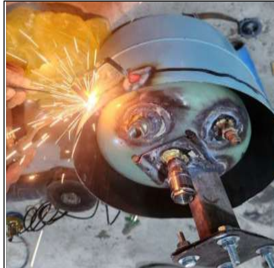
Figure 5: Lagging of the Reactor
